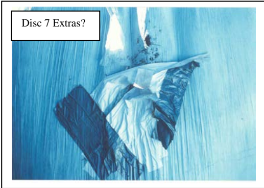
Figure 3. Plastic tape lifting due to poor preparation
